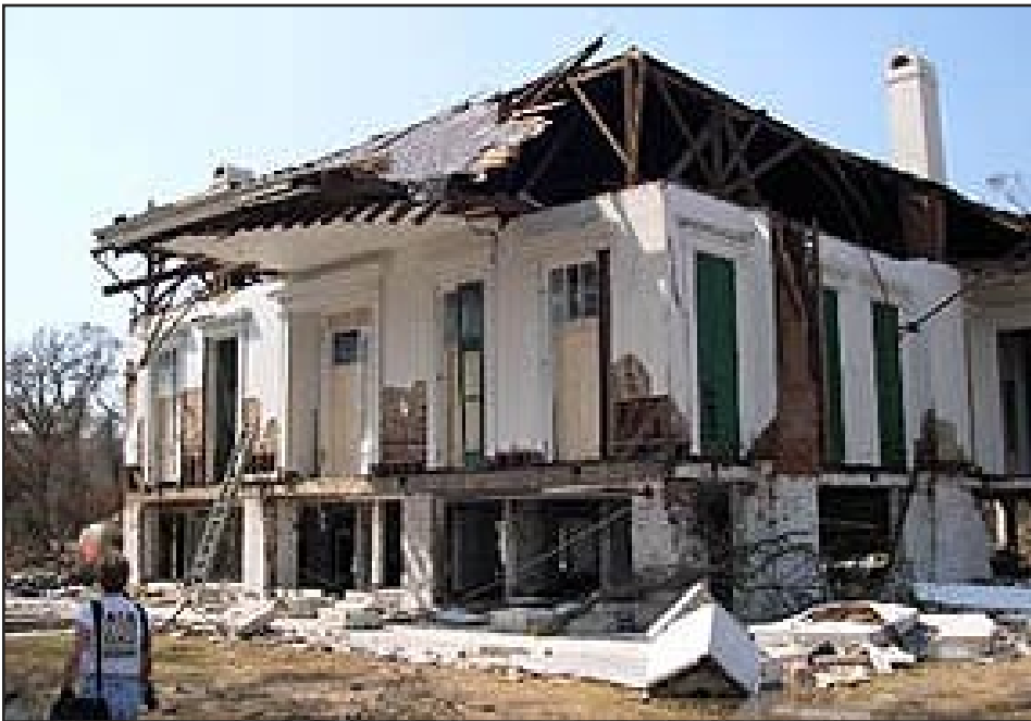
This photo shows the damage Hurricane Katrina wreaked on Beauvoir in August. As bad as the landmark was damaged, it fared better than nearly every other structure on the Mississippi coast.
